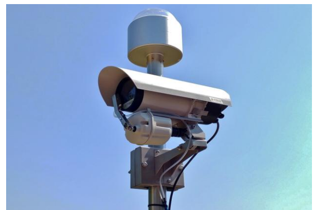
Tunnel entrance photometer FM-6
